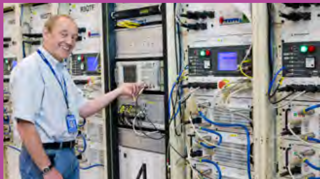
Right: Steve Gray making adjustments to the newly installed trim quad power supplies.
