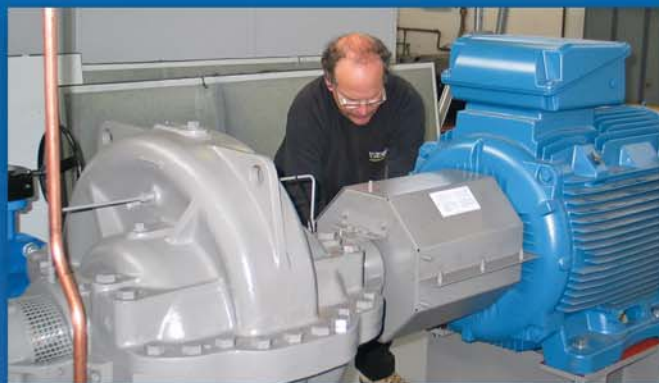
Right: Brian Hipwell working on one of the cooling water pump units.
