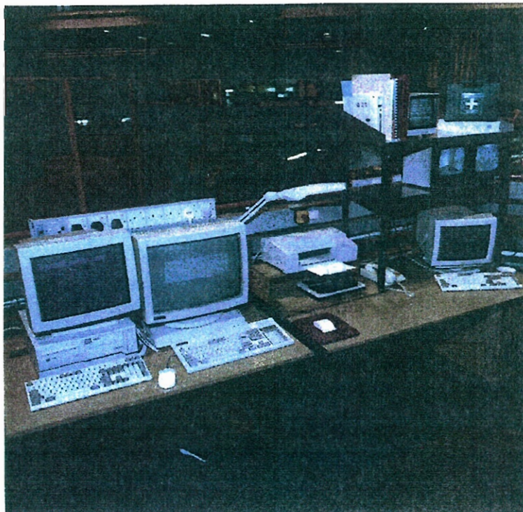
Fig. 3. Control centre on the gantry
