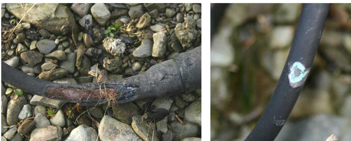
Figure 3: Examples of vermin damage to RG 213 cables.
