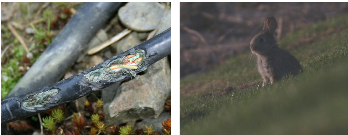
Figure 5: Examples of (left) a vermin-damaged relay control cable and (right) one of the probable culprits.
